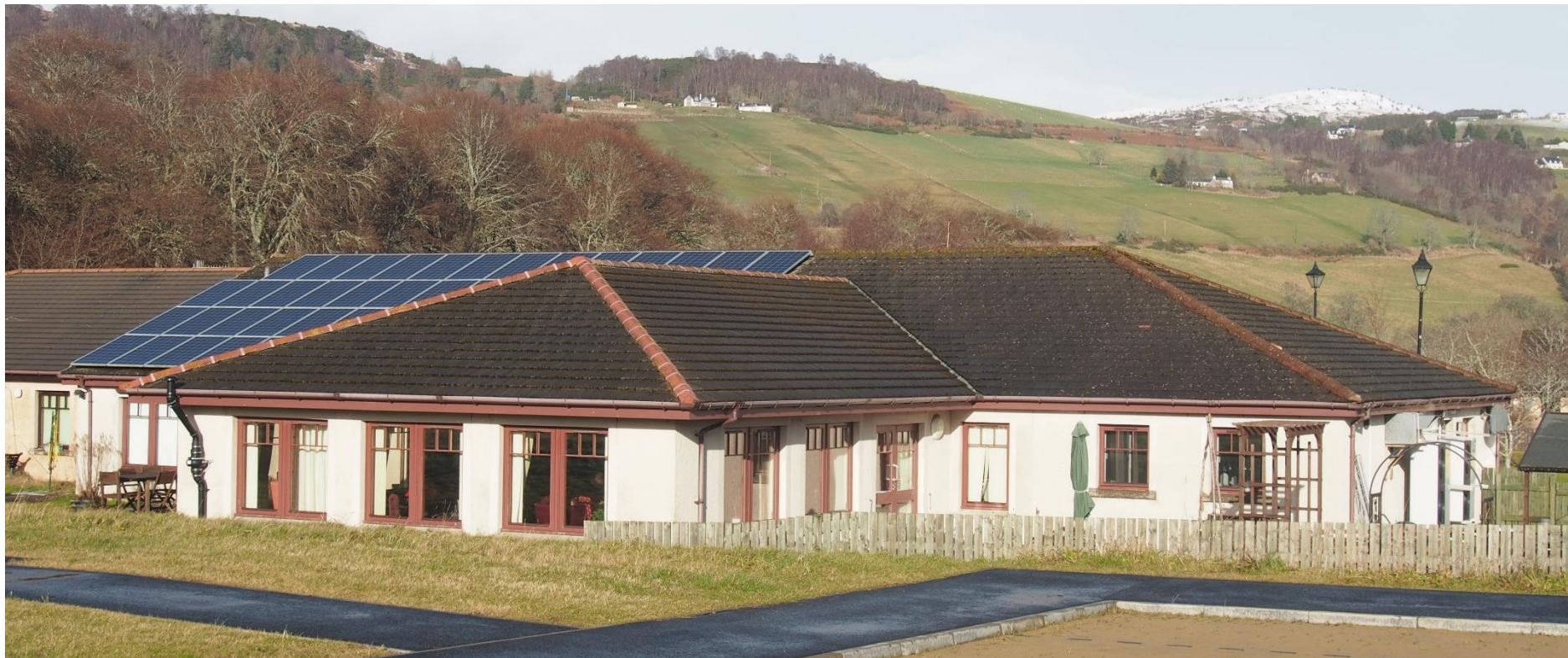
An 11kW solar PV array and two 12kW air source heat pumps provide low carbon power and heating to the community owned Glenurquhart Centre in Drumadrochit
