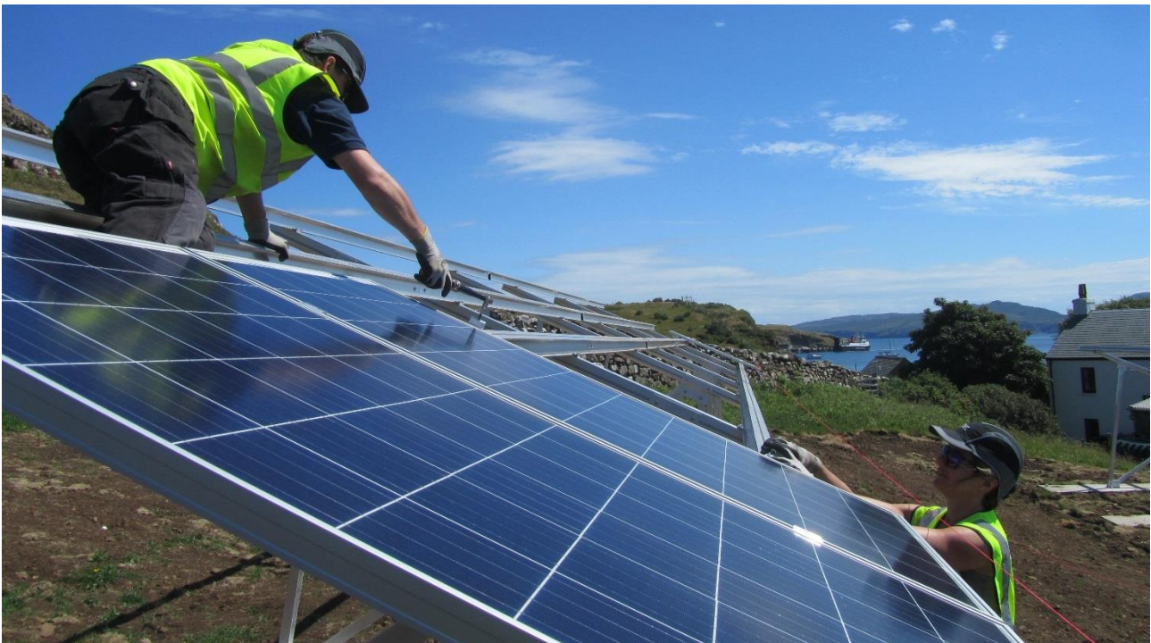
Installation of the 30kW solar PV array on Canna in 2018. It is estimated that the community owned renewable electricity system based on solar PV, wind, and battery storage will save 36,000 litres of diesel per year.
