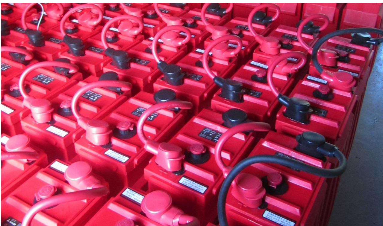
225kWh of battery storage has been installed on Canna as part of the community-owned renewable electricity system to provide continuous energy from solar PV and wind. Photo: Wind and Sun Ltd.
